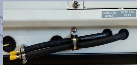
INPUT/OUTPUT FUEL PIPE
