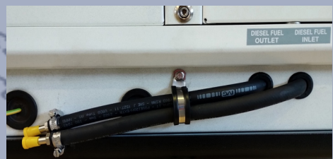
INPUT/OUTPUT FUEL PIPE
